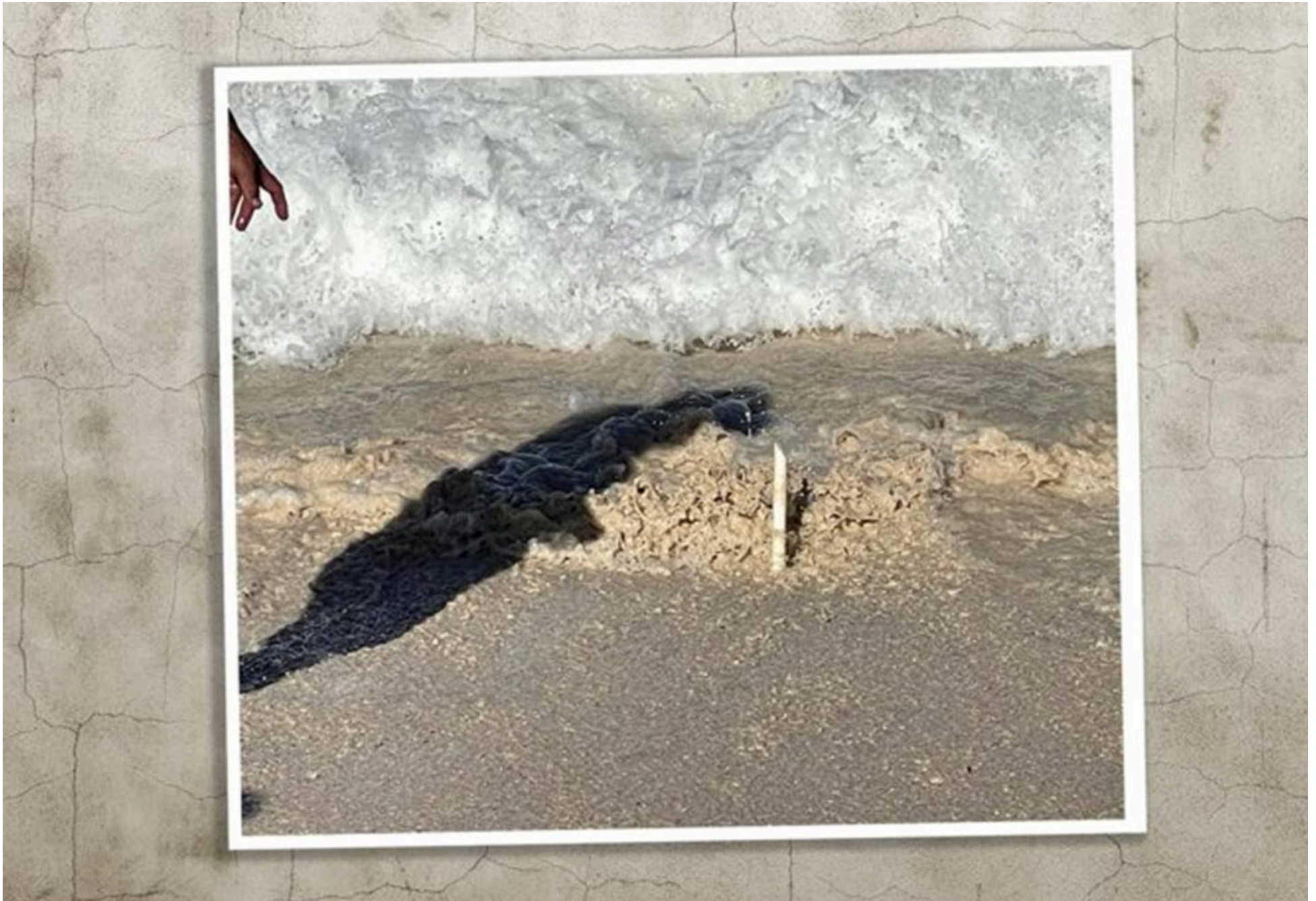
The electric sheath that emerges from the beach, opposite the Hôtel Cheval Blanc. Document Mediapart
