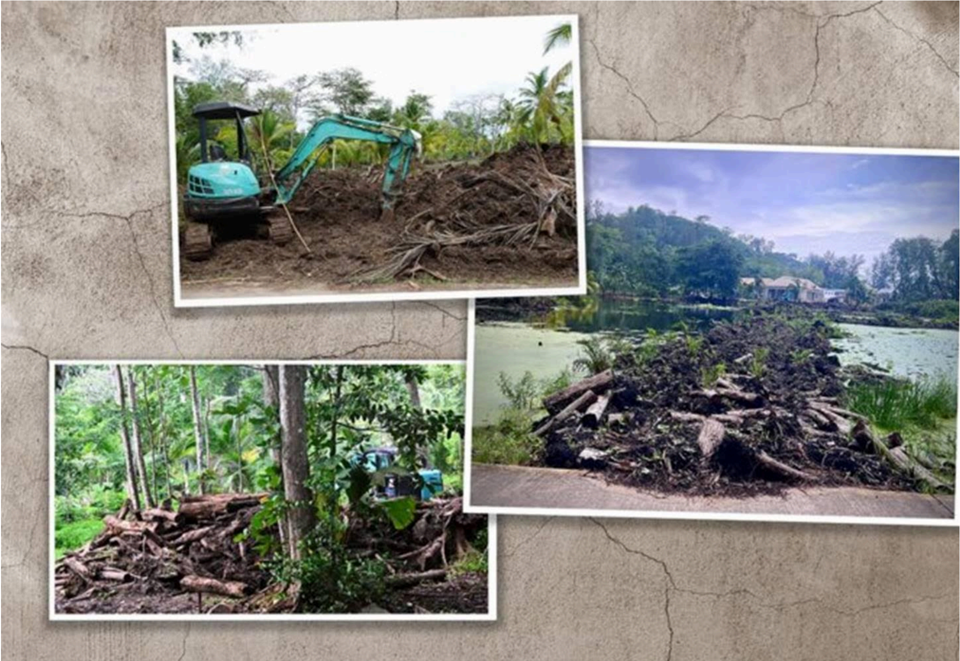
The work and the dyke (on the right) carried out in the wetland during the hotel's construction. - Mediapart/SBC documents
