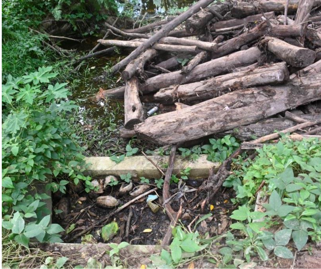
40a. A former sedimentation trap on outflow from wet land now totally clogged for three years
