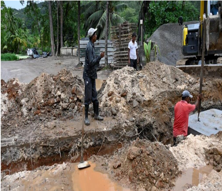
22a. Unexpected (and no notification) road trench
