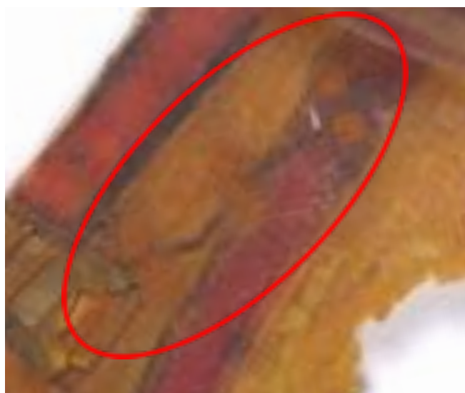
Figure 15. Corrosion associated with historic repairs near the loss on the leg, 2016. Image courtesy Amber Kehoe.
