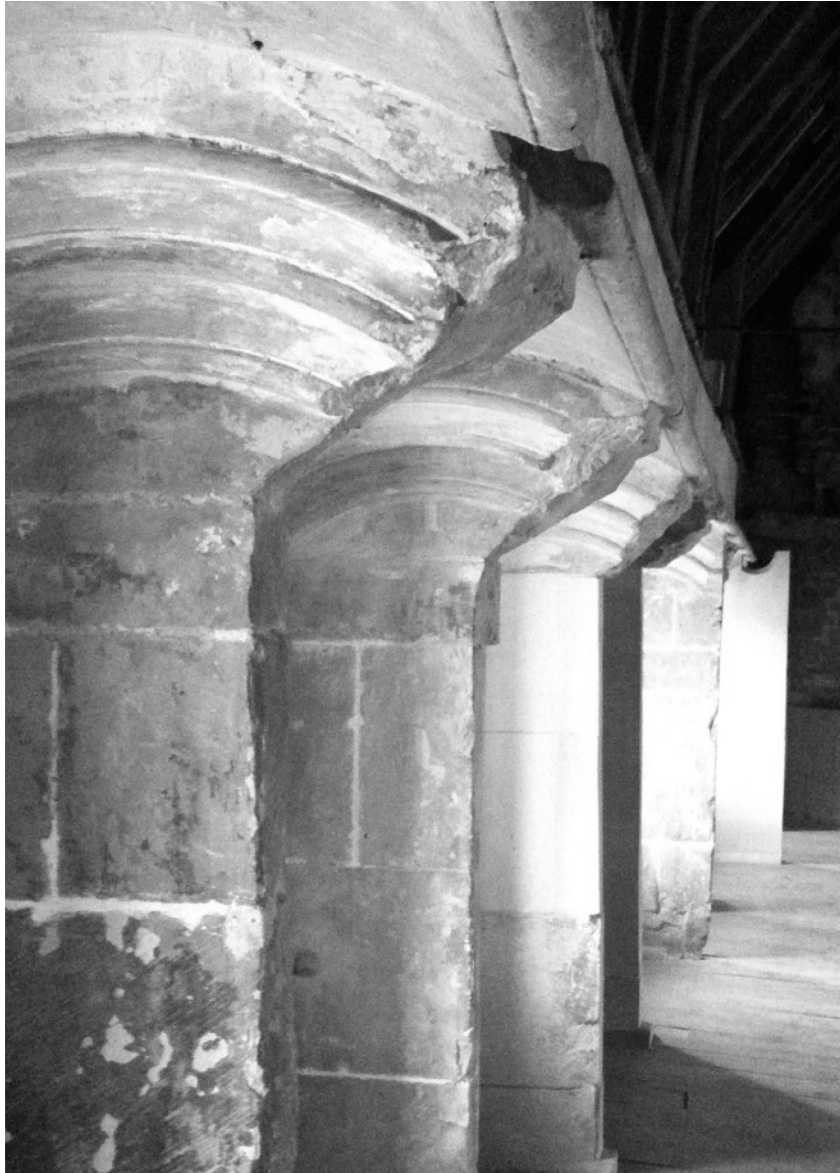
The curved stone arches have all been slashed, carving through the space to make way for machinery from a century before, the bow in the floor evidence of the weight that was once exerted upon it.
